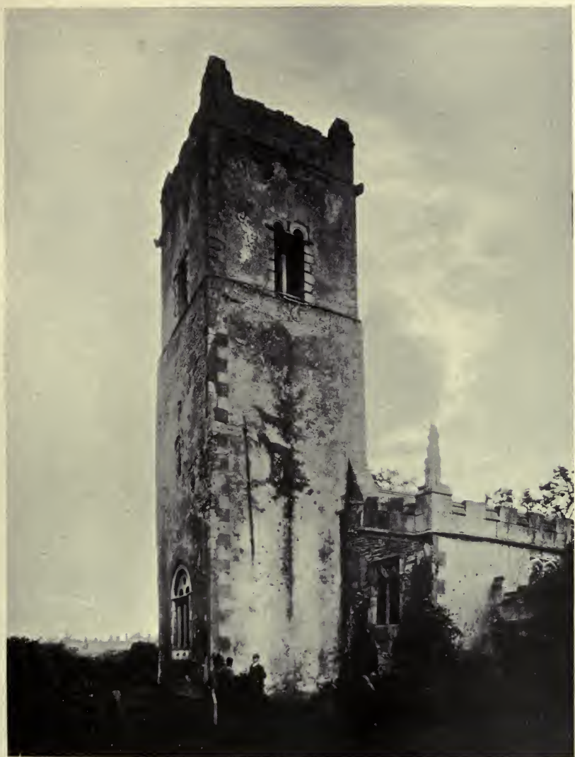
ST. MARGARET'S CHURCH TOWER, MARTON (BEFORE RESTORATION).
