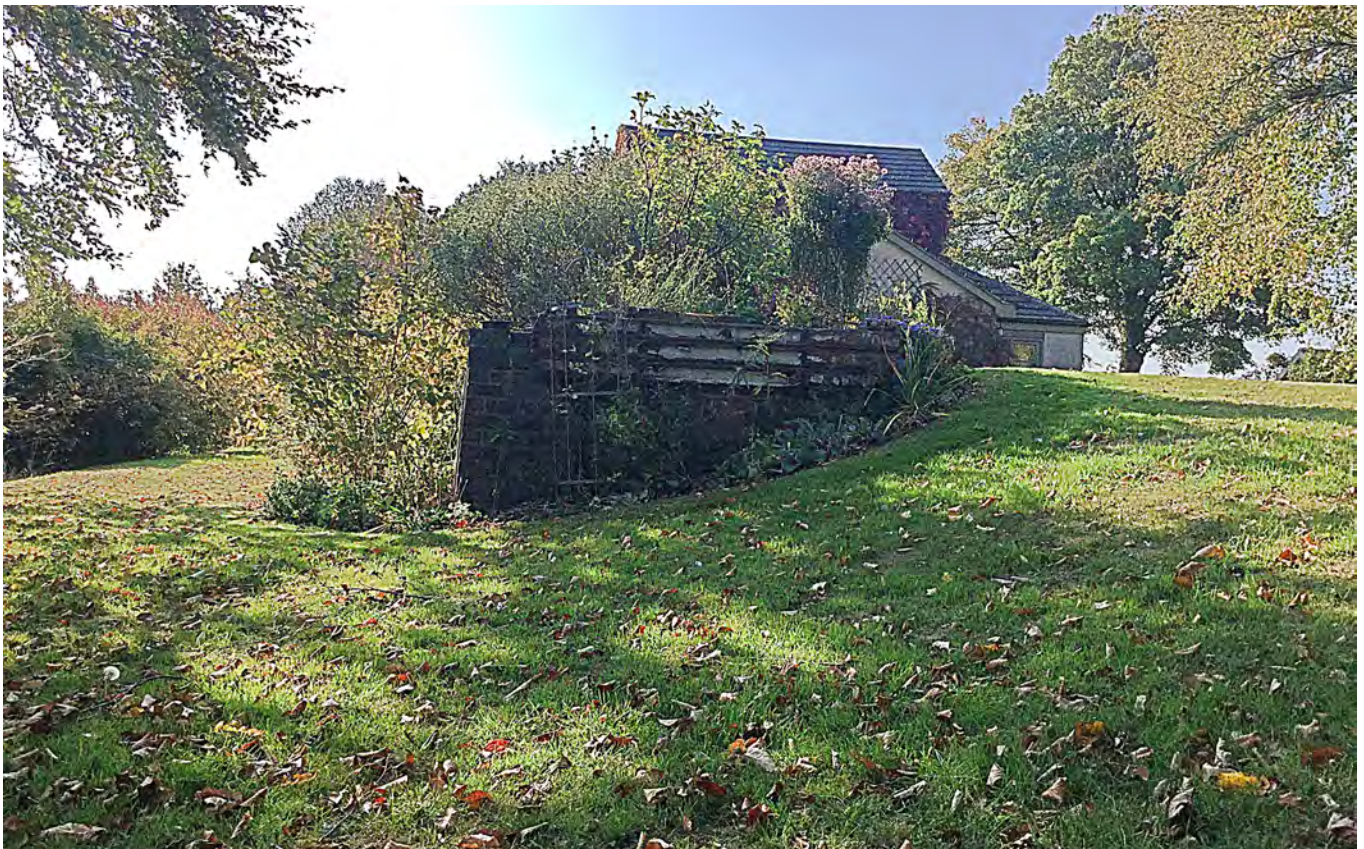
CATTLE RAMP WITH ORIGINAL 3 RAIL LENGTH BUFFERS STILL VISIBLE OCTOBER 2018 (PHOTO N.SPENCER)
